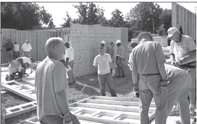
Volunteers raise exterior walls on the first day of the Millard Fuller Legacy Build, which was held Aug. 31 through Sept. 4 in Allendale.
