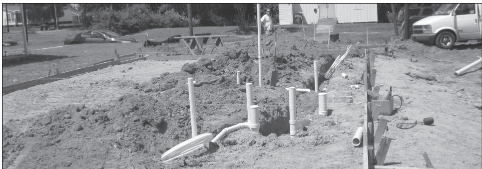
Building the houses begins with site work done before the Legacy Build late summer time frame.
